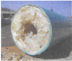
Above: Grease clogged pipe
